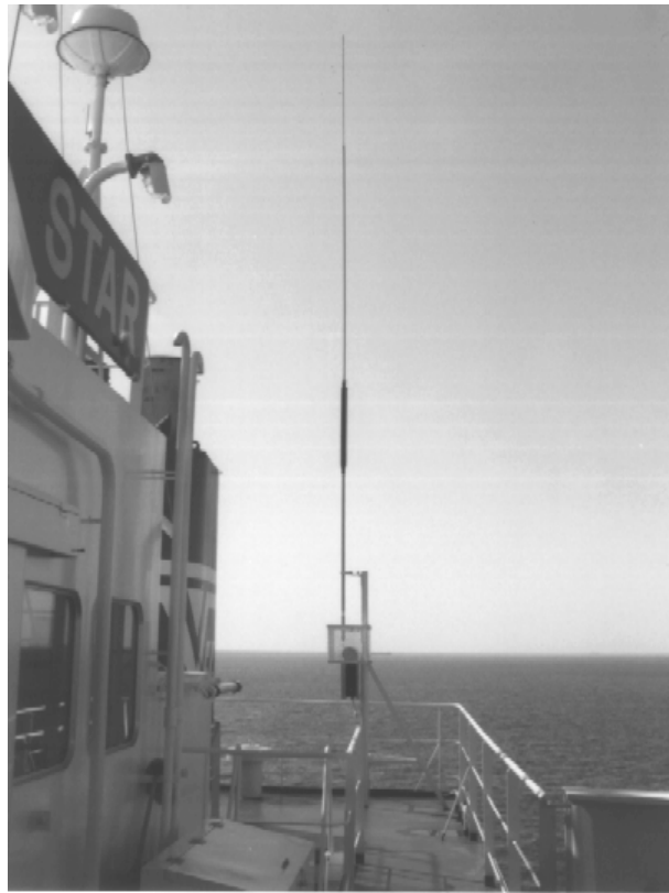
Actual DS410 Homing Beacon Installation
